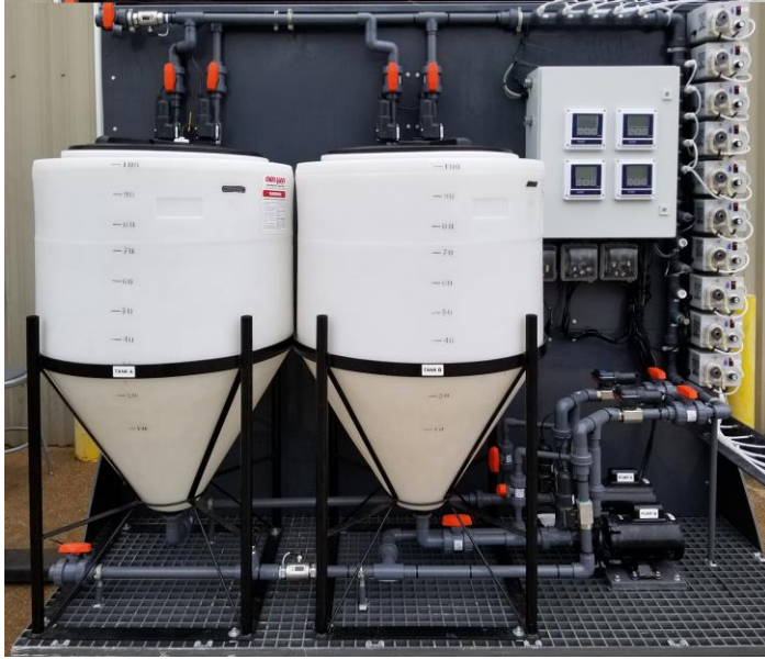
Total Grow panel consisting of two nutrient dosing reservoirs, each with a pH and conductivity sensor. The conductivity sensor is used to control the concentration of the nutrient solution.
